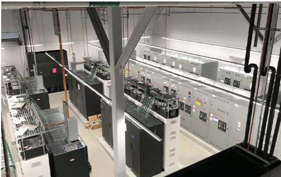
IMAGE 3: A room inside of a data center that contains UPS units, a critical part of a data center's redundancy.
